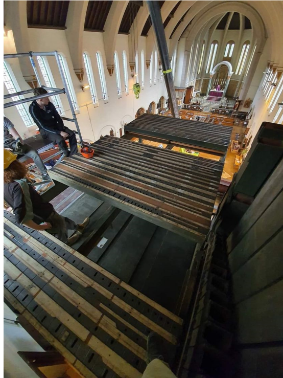
View of the nave from the organ gallery, where work is under way
